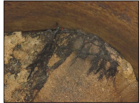
Cracked Bench with Roots (FM-08) 808-03
