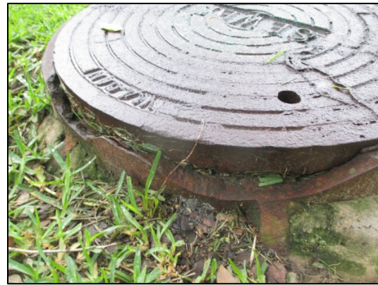
Broken Frame with Pick Hole Cover (FM-08) 828-01
