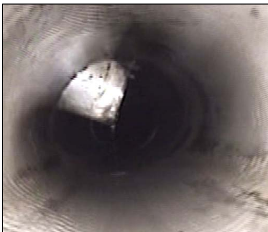
Service Break-Intruding at 141.7 ft. (FM-08) 6-16 - (FM-08) 5-16
