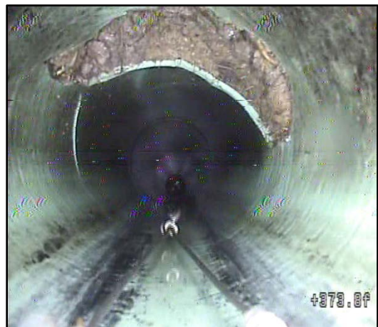
Pipe with Hole at 373.8 ft. (FM-08) 13-(FM-08) 12
