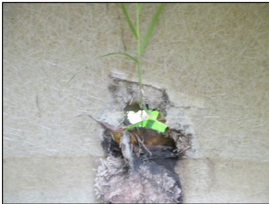
Hole in Manhole Wall (FM-08) 862-03
