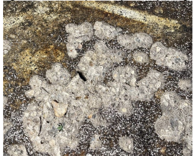
Figure 2: Close-up Example of Spalling
