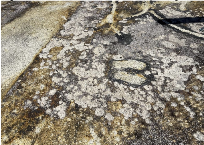
Figure 1: Fire Induced Concrete Spalling
