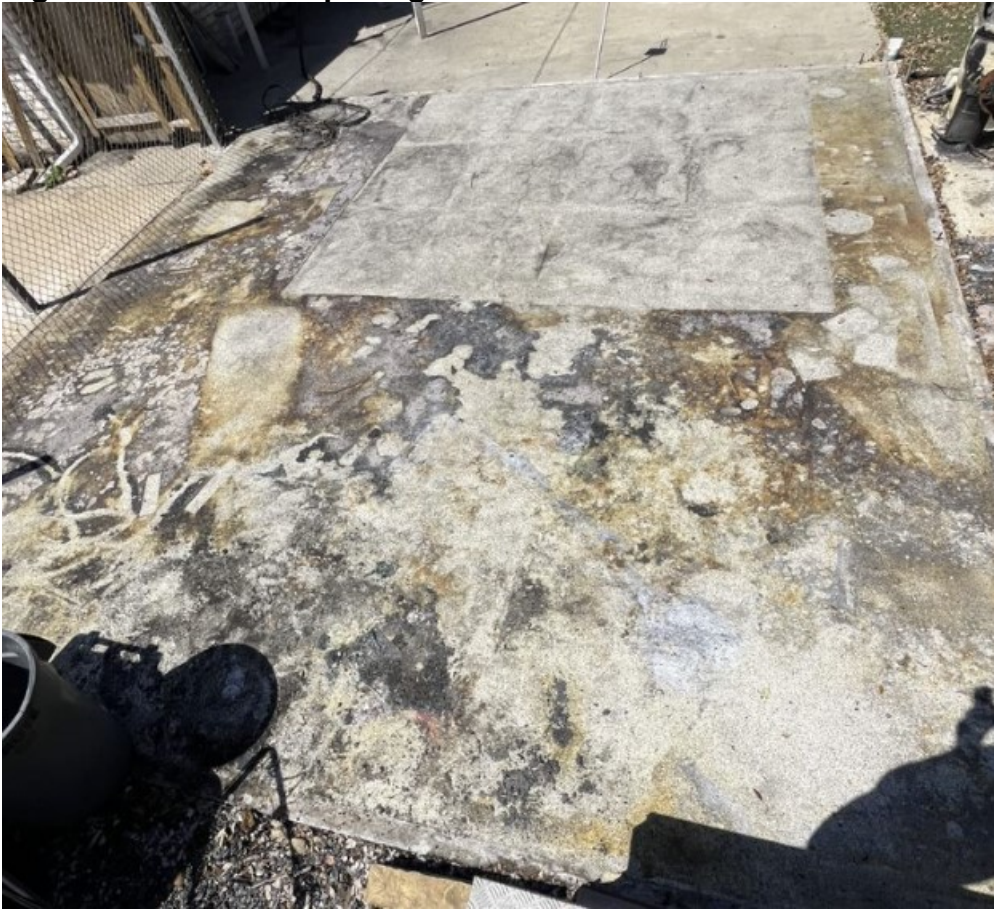
Figure 3: Concrete Spalling Present on Over 60% of the Structure
